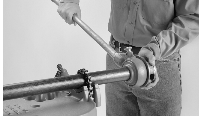
Figure 3 – Sliding Threader On Pipe
